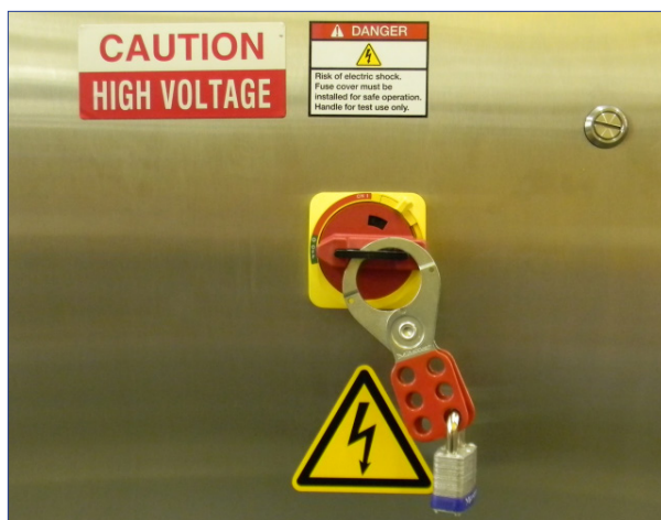
An example of a power switch lockout device.
